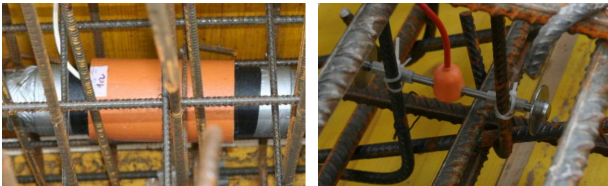
Fig. 3 EM transducer embedded on corrugated steel sheath (left)
